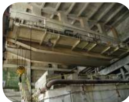
Gantry crane in a chemical facility was mechanically abraded and coated with Resichem 501 CRSG
