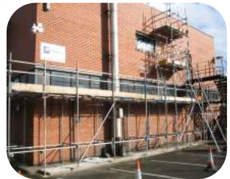
Training facility in the UK was refurbished using Resimac corrosion protection systems. All surfaces were mechanically abraded and primed with 506 Aluprime and top coated with 508 UVPU
